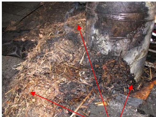
Bird nest inside chimney
