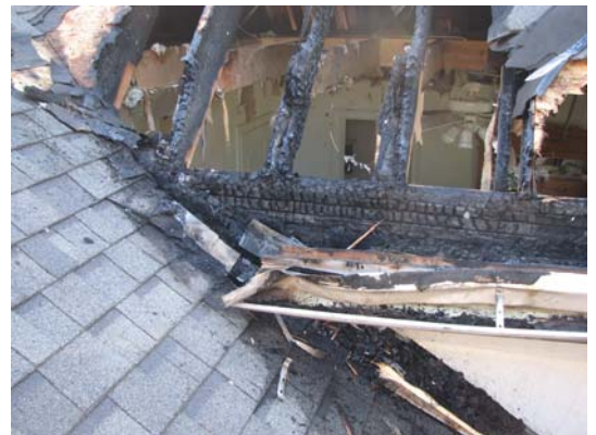
2 nd Exposure – Embers dropped down onto pine needles in the gutter of this single family home.
